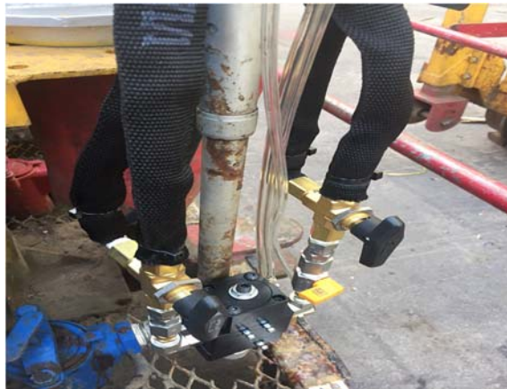
Nylon Protective Hose Material Added At Dispensing Valve
